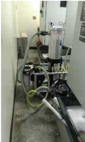
Pump/filter unit cleaning machine sump. (Model shown with optional cartridge filters on pump discharge.)
