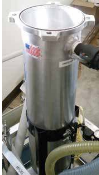
Pump/filter unit open for service.
